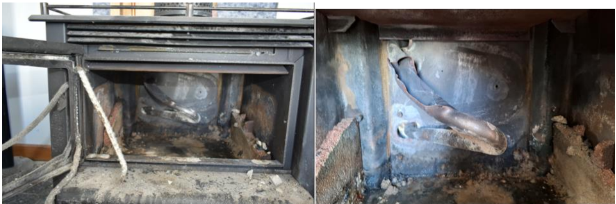
A capped off flow and return from a water jacket in a wood heater that has exploded; causing serious injury
