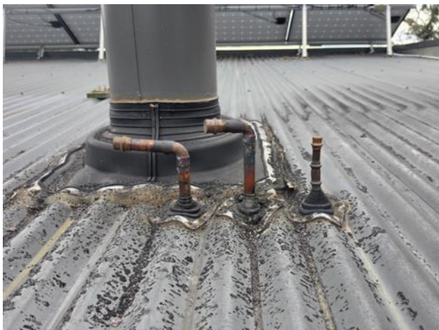
Sealed off flow and return pipework
