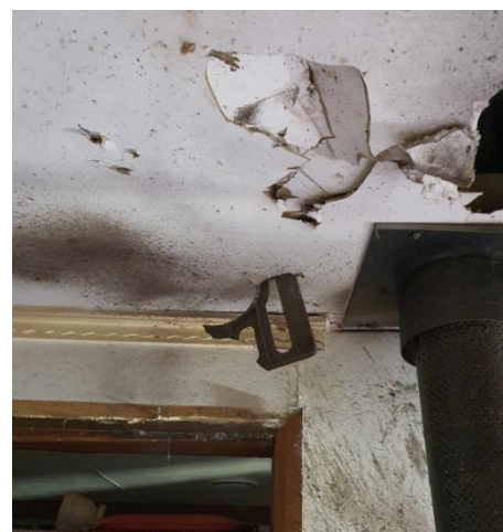
A large fragment of cast iron lodged in a ceiling
